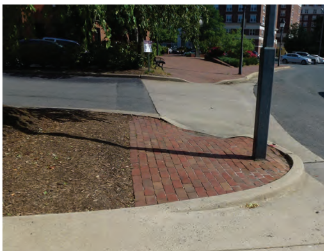
Missing and non-ADA compliant curb ramps
