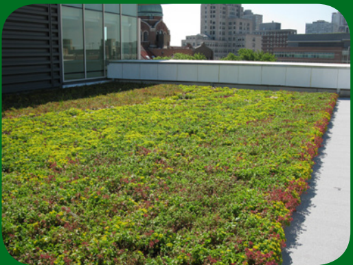
Green roof, Loyola University, Chicago, IL
