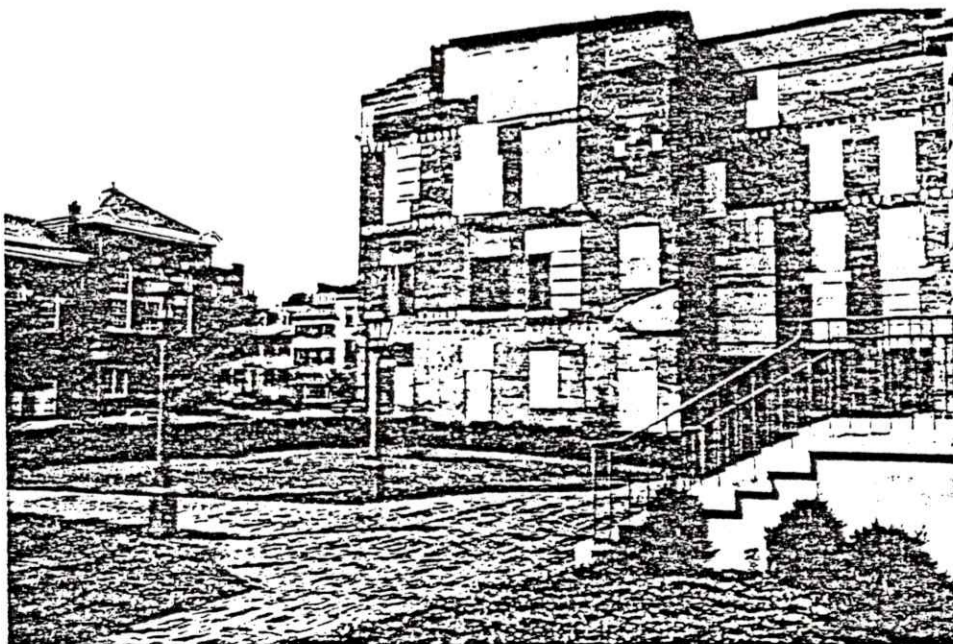
VIEW OF SOUTH ELEVATION. NOTE DETERIORATED CONDITION OF EXTERIOR WALLS.
