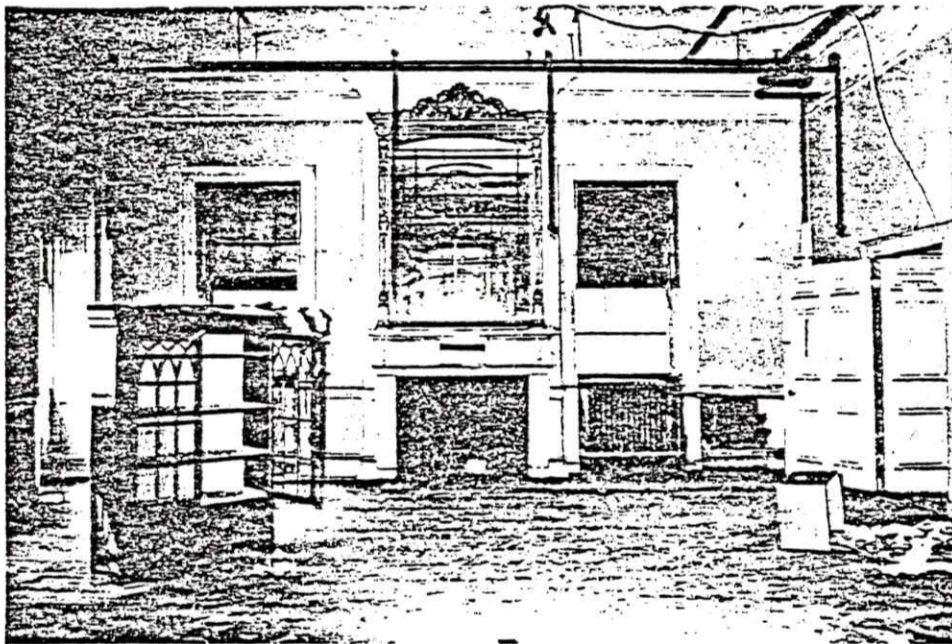
PHOTO OF MAIN LOBBY. NOTE INADEQUATE LIGHTING, DETERIORATED WALLS AND CEILING, AND EXPOSED PLUMBING.
